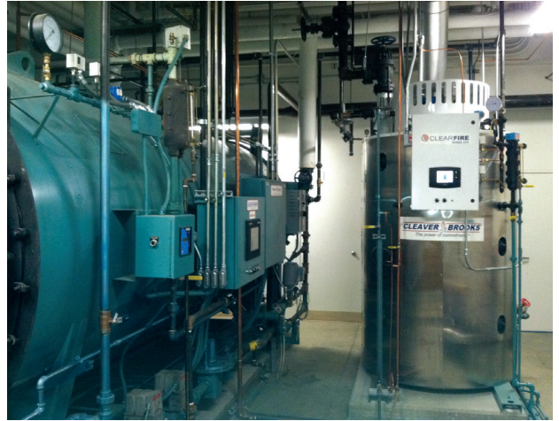
Logan Regional Hospital paired a 60-hp boiler with its existing 300-hp boilers. The new system has helped the hospital reduce operating costs by 30 to 40 percent.
